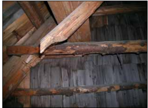
12. Presence of using the un-barked elements in the roof construction, Church Prašivá
