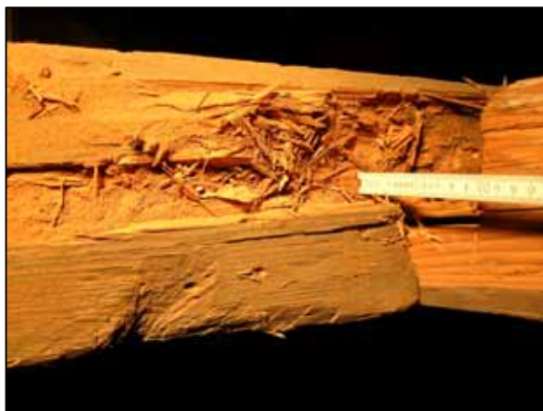
7. Surface damage by wood attack insects, 50 mm depth, Church Prašivá
