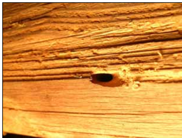
8. Typical oval emergence hole from the longhorn beetle ( Hylotrupes bajulus ), Church Prašivá
