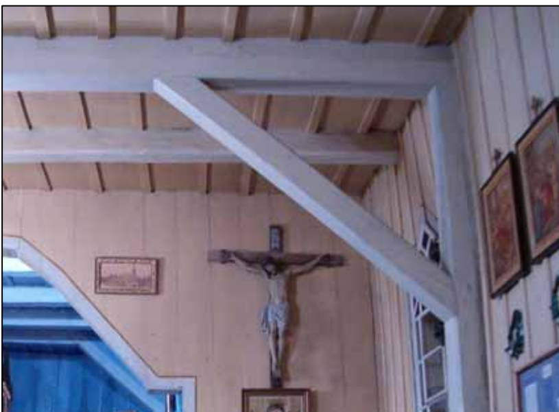
23. Joist ceiling is supported by walls and columns with struts. Beams are also members of roof structure. Several beams are doubled.
