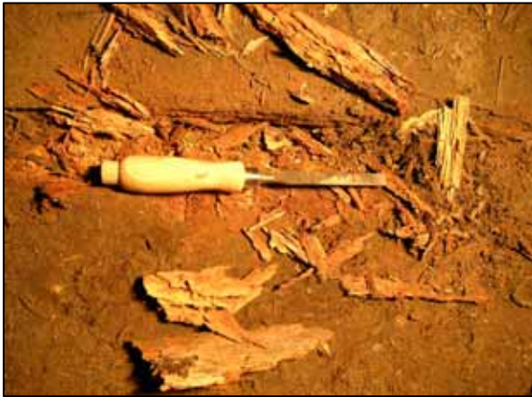
11. Damage of decking of ceiling by insects, Church Prašivá
