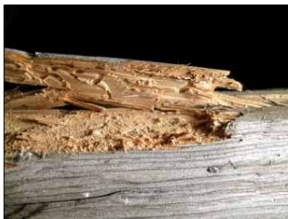
10. Wood damage on surface by insects, existing the bore dust, tunnels, Church Prašivá
